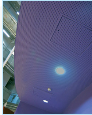
Profab access panel into Rigitone ceiling at the Curve Performing Arts Centre Leicester
